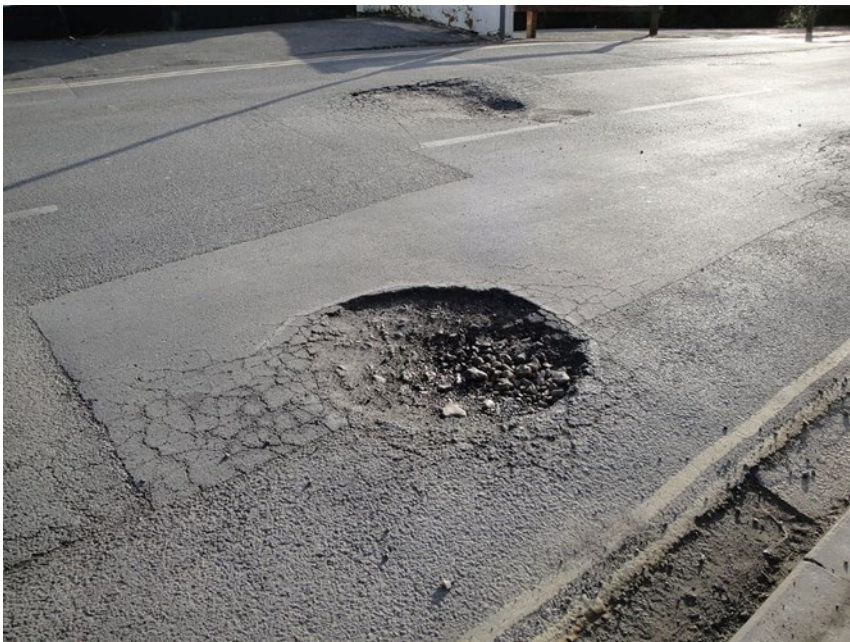
Figure 3: Potholes on asphalt pavement
