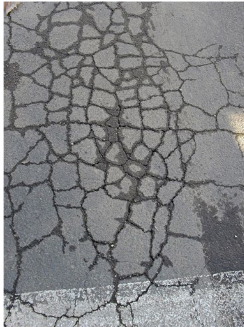
Figure 2: Low-Temperature Cracks (LTCs) on the asphalt pavement
